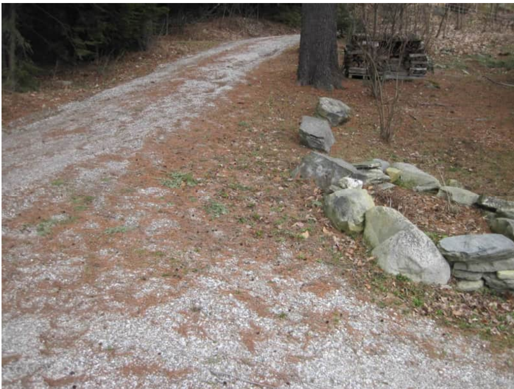
Figure 56: Project 49 – East Shore Lane rain garden
