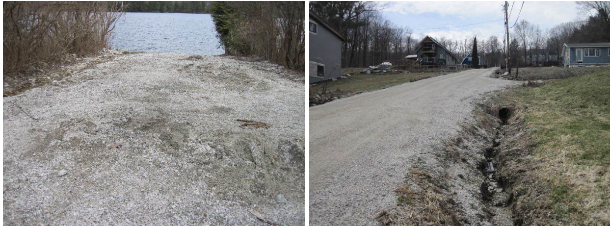
Figure 4. Stormwater from Shadow Lane flows into Lake Iroquois
